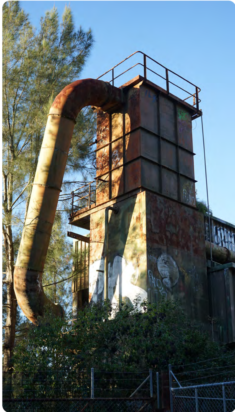
Existing Crusher Plant
