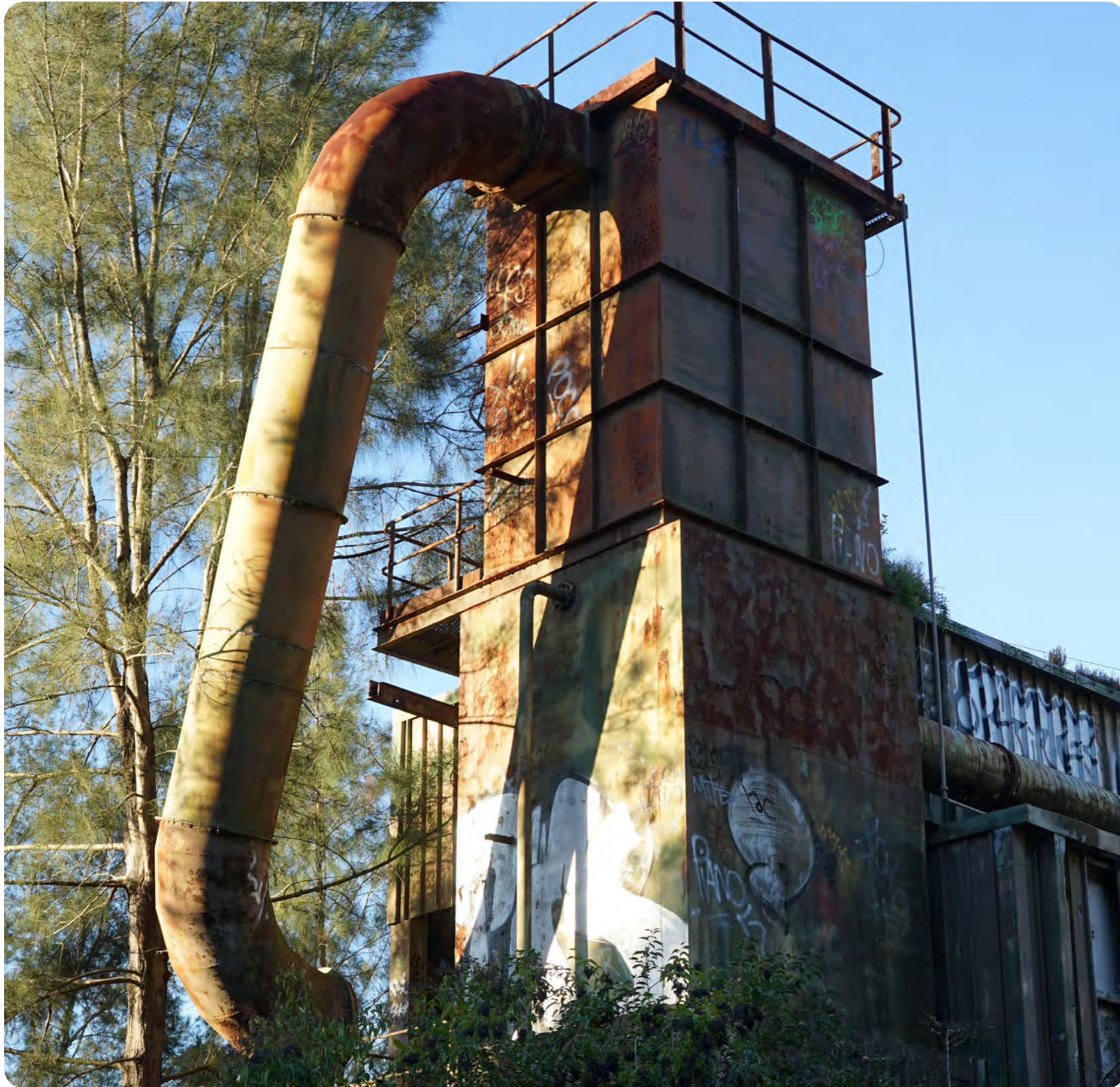
Existing Crusher Plant
