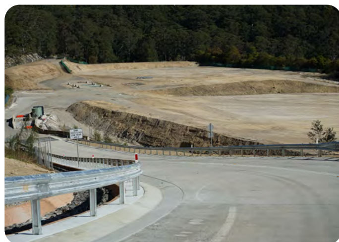
Existing steep vehicle access into OMV from Peats Ferry Road via Bridge Road
