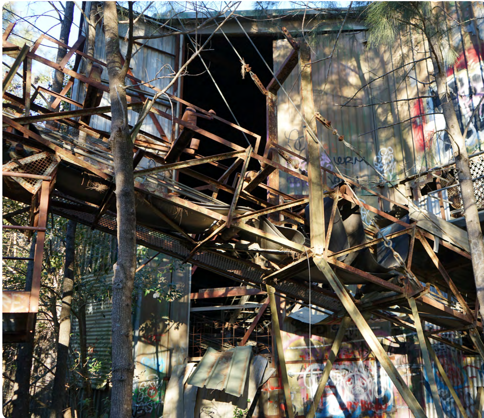
Existing Crusher Plant
