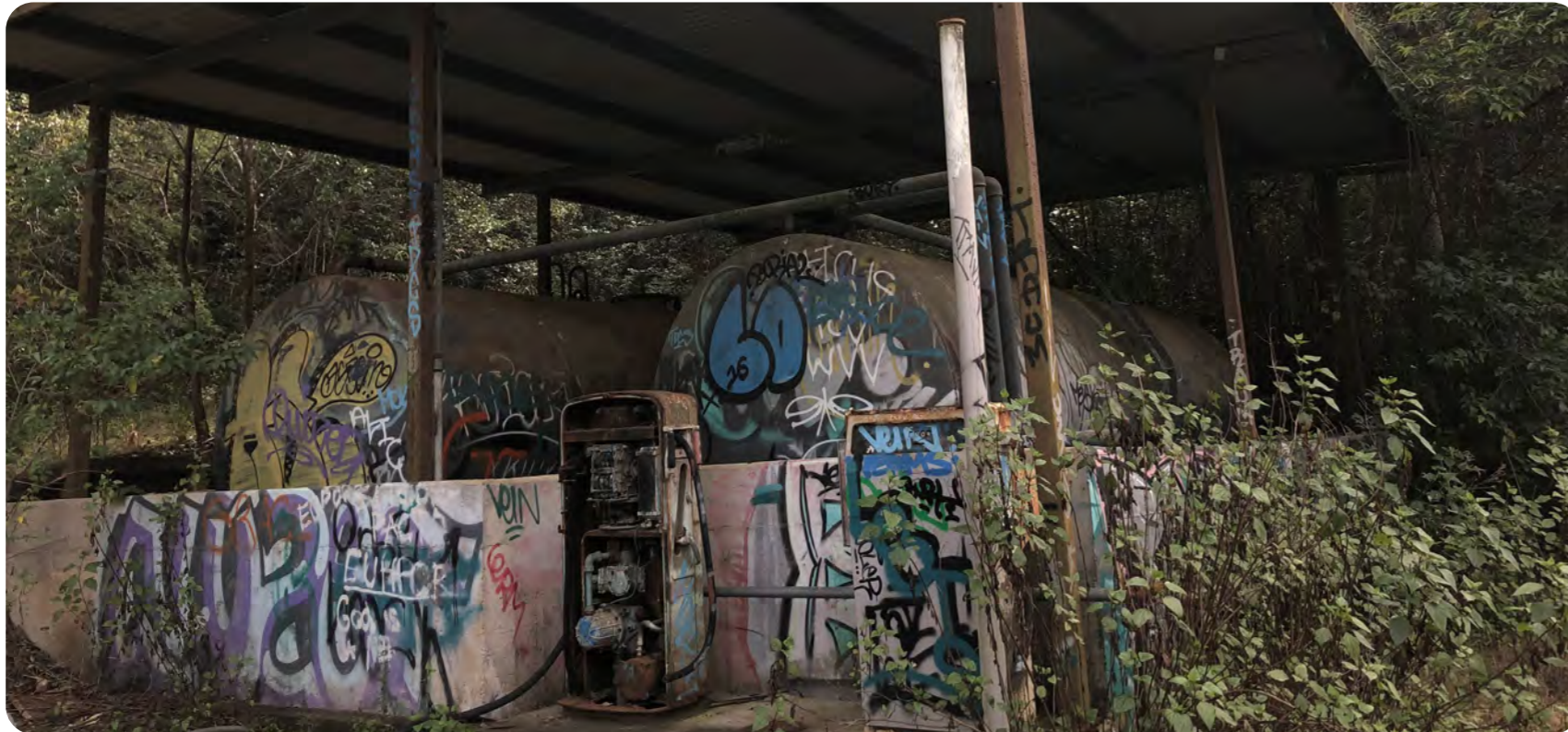
Fuel storage tanks
